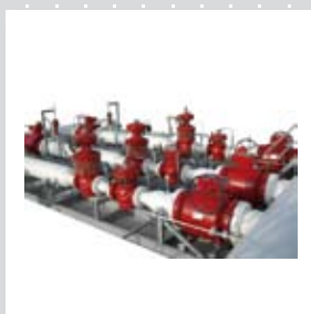
Reducing & metering station
